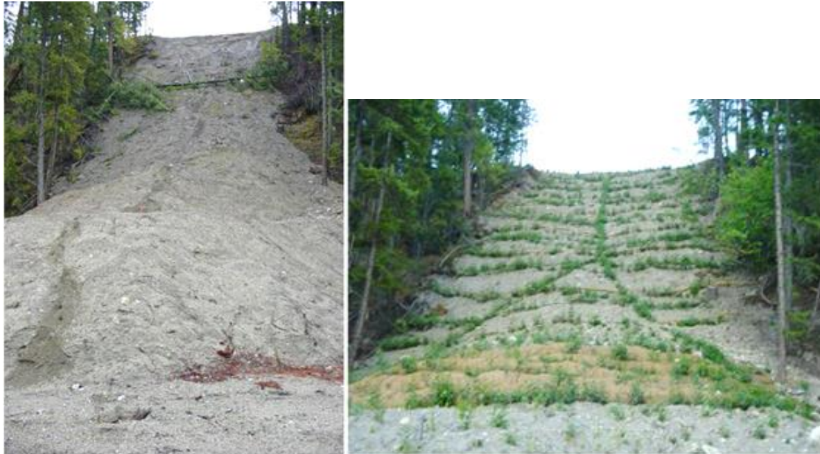
Figure 42: Diverted drainage in a case-study in Southeast British Columbia, Canada, caused by a landslide in February 2002 (left). In March 2003 (right), live pole drains systems (i.e. cylindrical bundles made of live fascines with desirable rooting properties, used as a collector drain in conjunction with lateral drain fascines installed in a chevron pattern) were installed to address underground seepage rising into the upper third of the slope. Vegetated lifts, brush layers, fascines and live staking (planting of live poles) were installed at the same period. Note that this example represents an application of a set of different NBS in the attempt to control a mass failure process. source: (Stokes et al., 2014).
