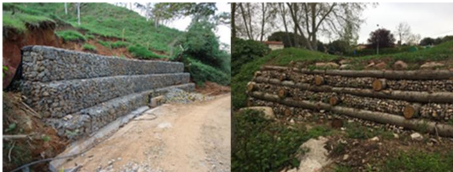
Figure 6: Slope stabilisation with classical methods (gabion) (left) and with bioengineering techniques (right) (Cribwall Krainer).
